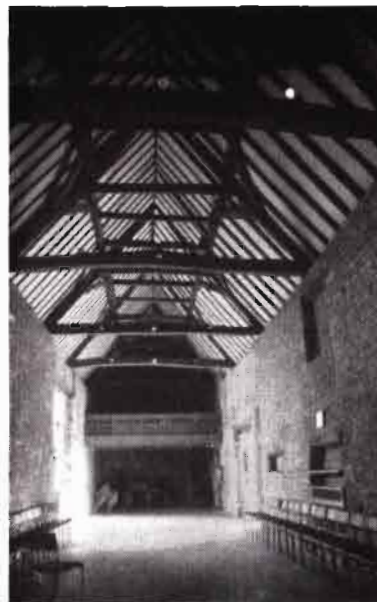
Warsop Parish Centre—Barn Conversion, November, 1977. The Trust grant aided the sympathetic conversion of this building from a barn to a Parish Hall and has since had the pleasure of holding its Annual General Meeting in this delightful building.
