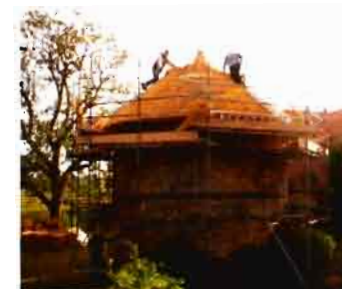
Above: Rethatching in November 2011 by the team from Roger Scanlan Thatching of Northampton
